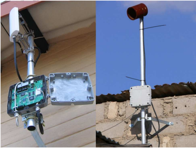
Fig. 3. Outdoor mesh node with repackaged Linksys WRT54G electronics in a waterproof aluminium case. The picture on the left shows an installation at node D is using a commercial 8dBi flat panel, the picture on the right shows an installation at node H which is using a home made Cantenna
